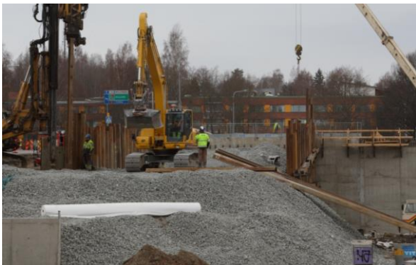
Figure 2. Up to 8 m high FGA embankment between sheet pile walls during bridge construction worksite at E12 highway (Auvinen et al. 2013).
