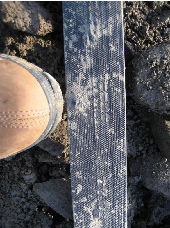
Figure 8 Minor damage to reinforcement.
