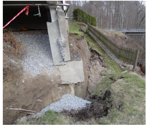
Figure 3 Backscarp of the landslide restricted by the pile foundation. Concrete pile supporting the corner foundation visible.
