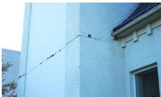
Figure 5 The crack in the Bell tower.
