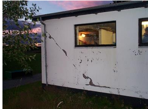
Figure 6: Damaged squat wall in Hveragerði after the 2000 earthquake with visible shear crack.
