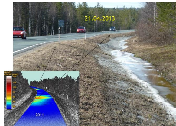
Figure 6. Laser scanner data based frost heave analysis from HW4 in Finland. The ditch is filled with ice and in the summer the bottom of the ditch is 60 cm deeper than the ice surface.
